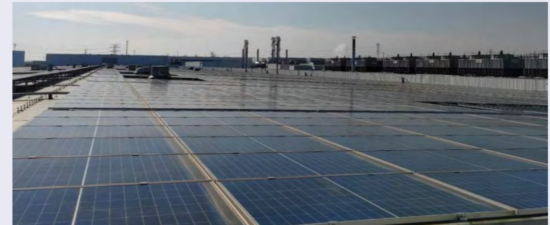
Rooftop PV Power Plant
